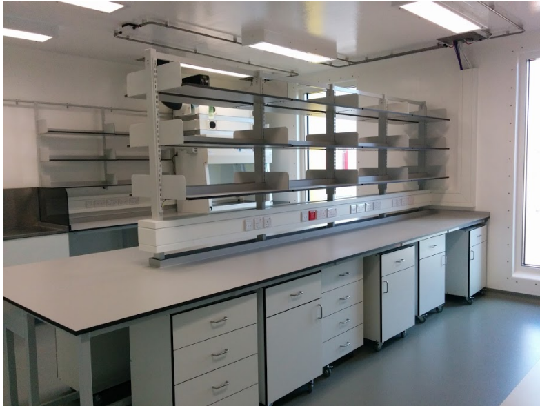
Limited Network sockets
